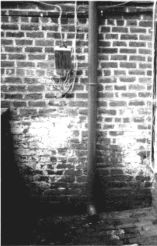
Areaway at the northwest corner of the pavilion with surface-mounted wiring, improper pointing, and open joints in the paving
