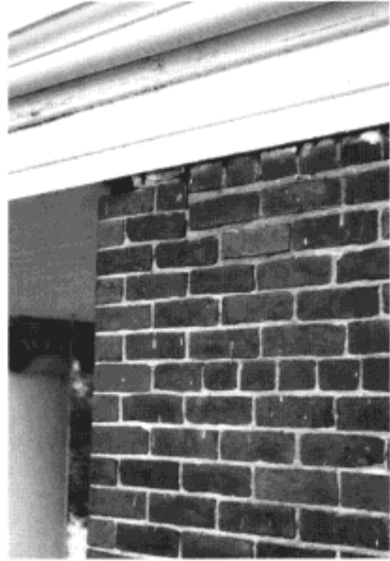
Improper pointing and open mortar joints at the east end of the north elevation
