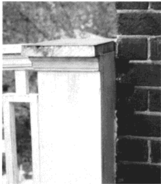
Broken brick at the west end of the south roof terrace
